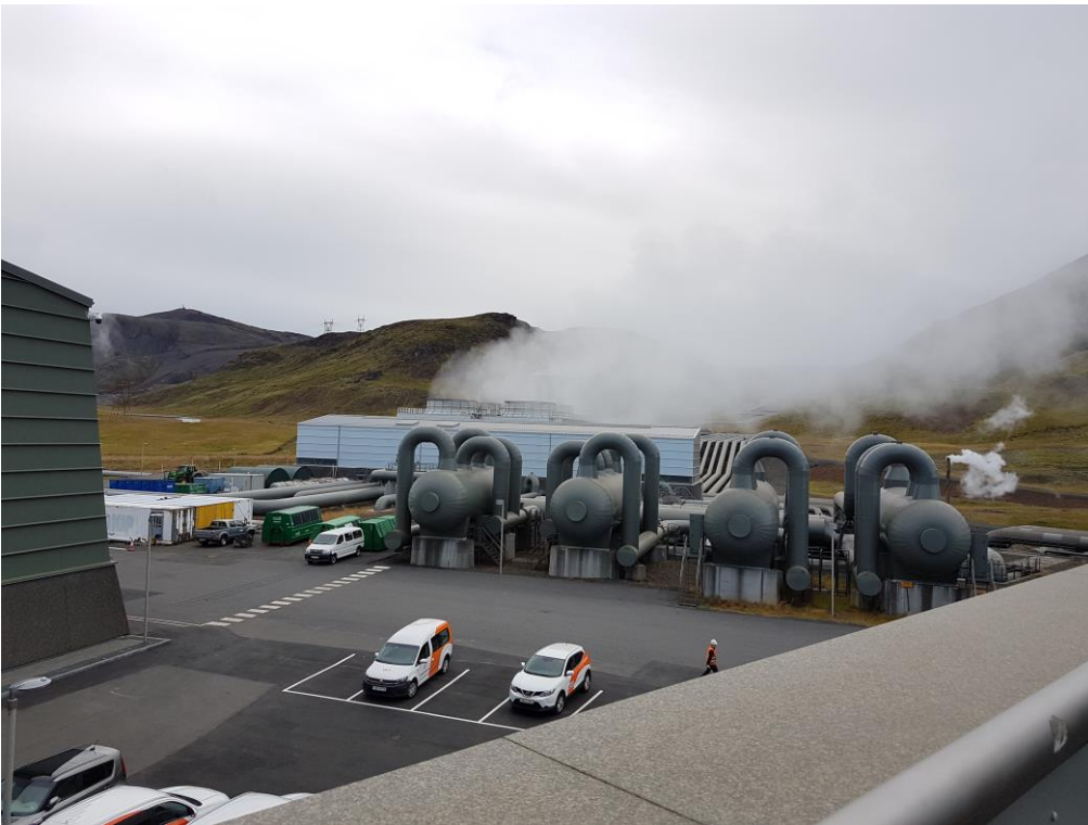
Power plant – utilities at the back site.
